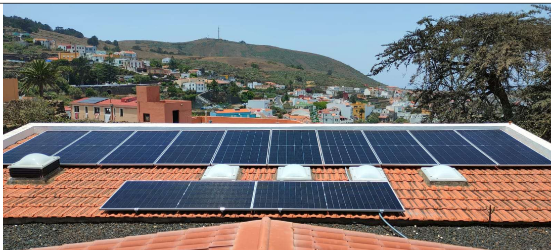
12 placas fotovoltaicas 605 Wp = 7260 Wp
